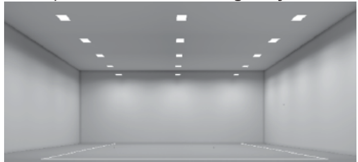
C) Fluorescent T5 HO high-bay
